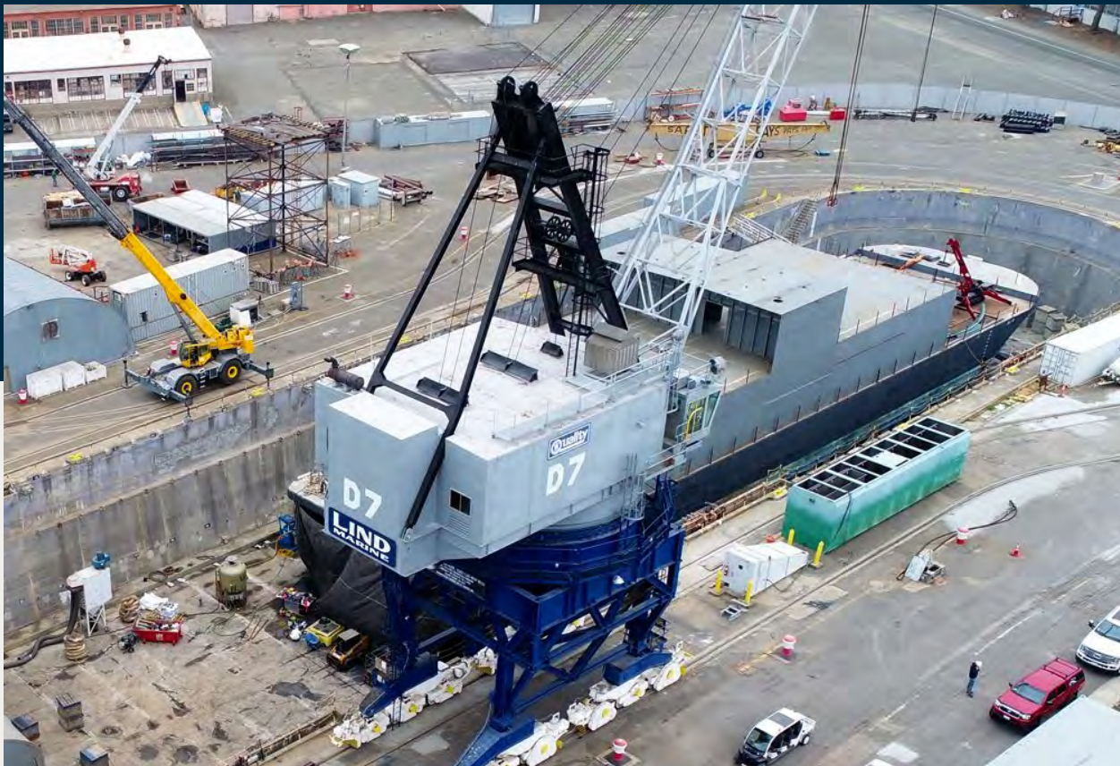
Lind Marine Completes Waterborne Data Center Barge Project on the Mare Island Naval Complex in Vallejo, CA
